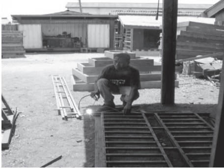
Plate 1: Welder without protective goggles Photo credit: Akorsu (2010)
